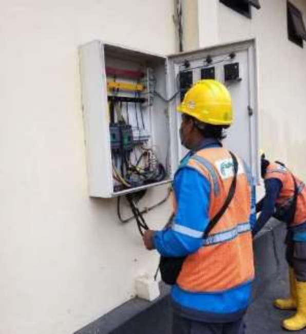
Connecting distribution panel
